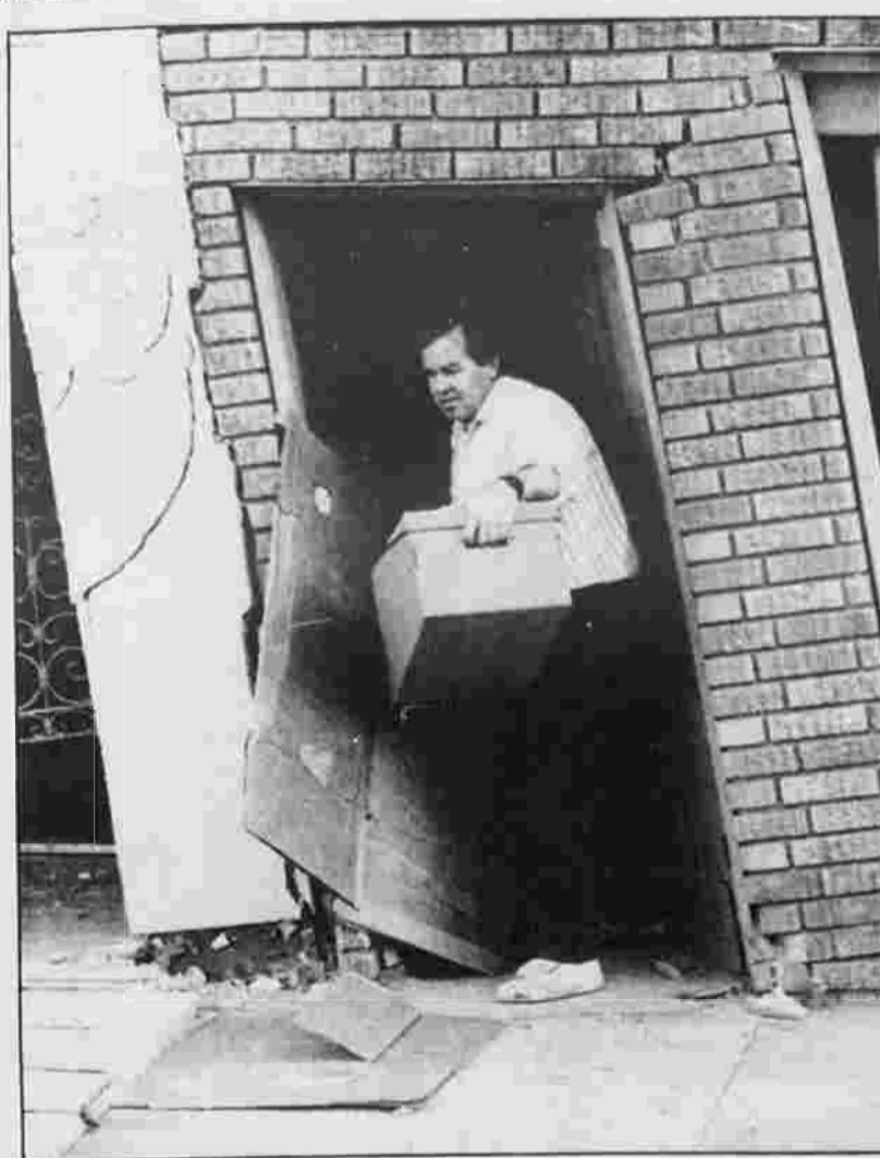
TILTED HOUSE — A man carries a box through a tilted doorway in the Marina district of San Francisco Thursday.
